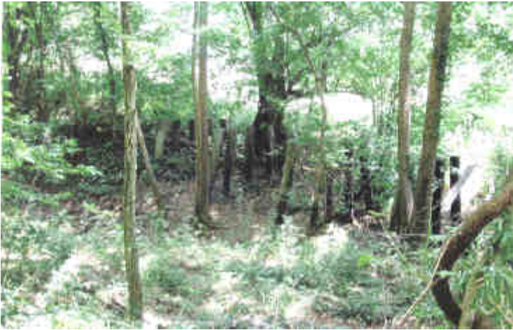
Trestle Remains (200.2), looking east – This same trestle was photographed by Leonard Sherman in the early 1970's (the mile location is from his notes), when some of the caps and traces of stringers remained. The large tree just beyond the pilings in the center appears to be three or four feet in diameter. In Leonard's photo, it looked smaller than the pilings and most of the other trees did not appear to be present at all.
