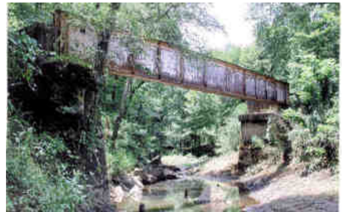
Lost Creek Bridge (205.6), looking southwest – Only the near side 60-foot girder remained; the other was "pouched" years ago. Crossed pile trestle approaches (photo 27' piers) south and two 12' piers) north) doubled the overall length of the bridge, which was 19 feet high. (Bridge details based on notes by Leonard Sherman)
