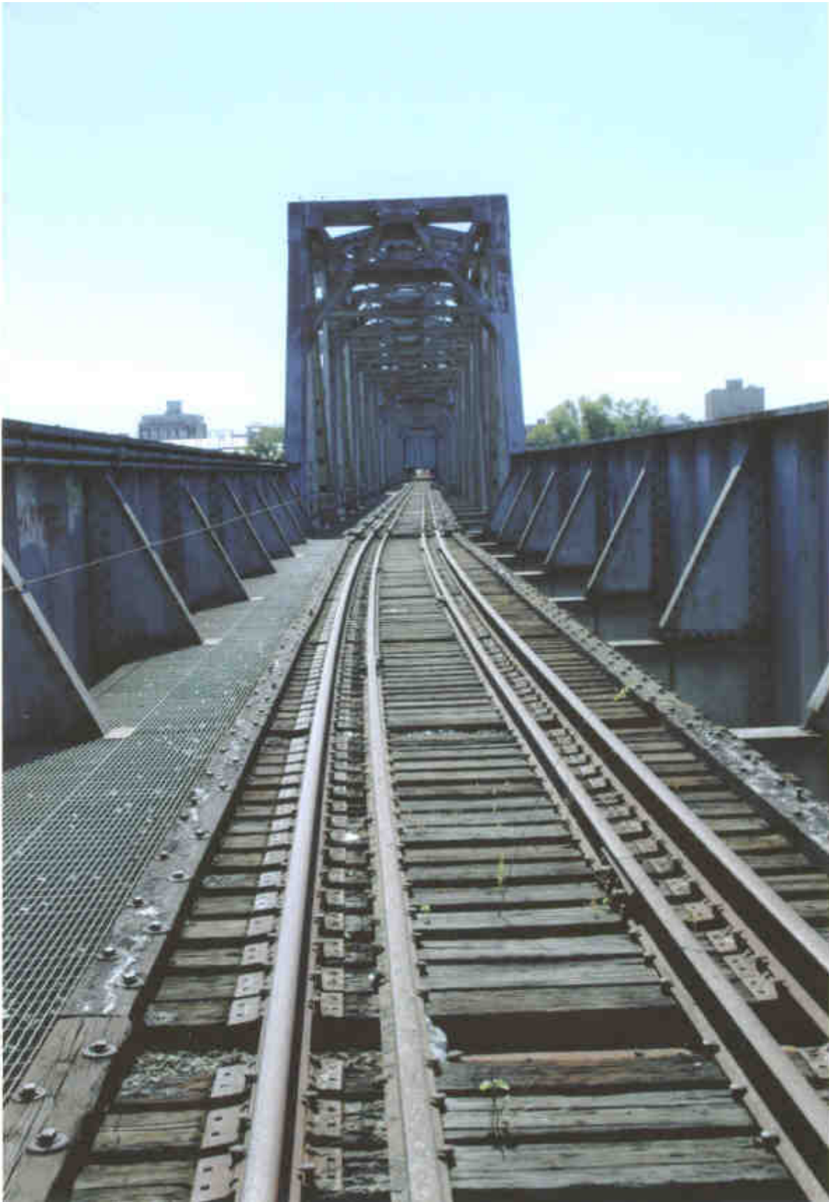
The abandoned Missouri Pacific Junction Bridge over the Arkansas River between Little Rock and North Little Rock will soon become a pedestrian walkway between the two cities. Union Pacific gave it to the city of Little Rock in 2001. Work has begun on the conversion - no track remains outside the bridge. ( John C. Jones photo, November 2005 )
